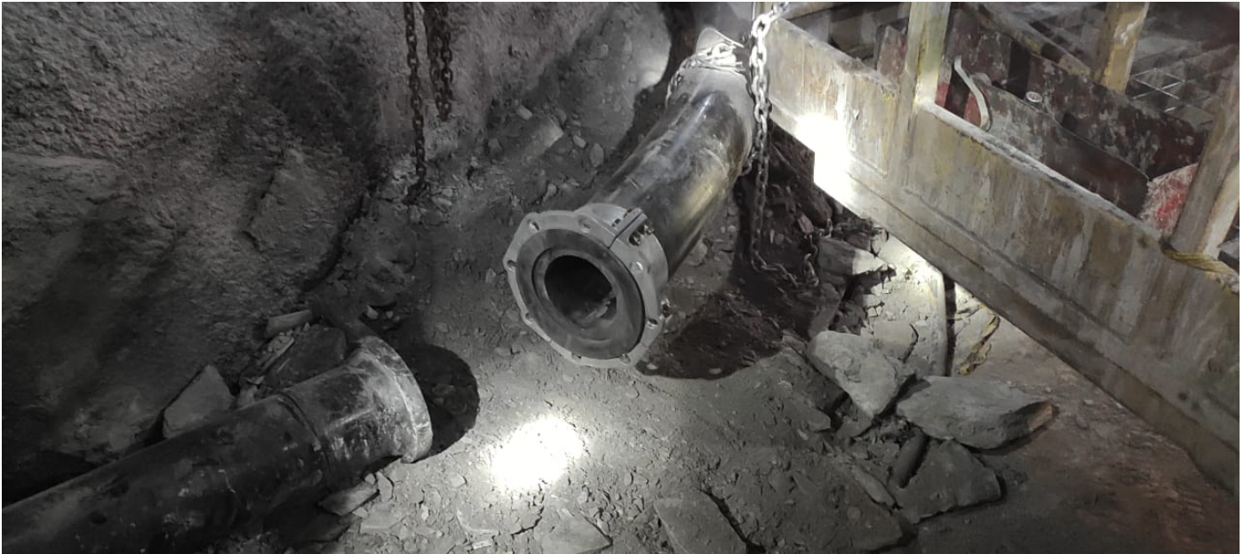
Pexgol pipe to transport effluents at 30°C / 86°F in an underground mine.
