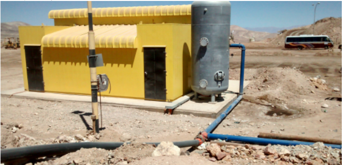
Air compressor system
