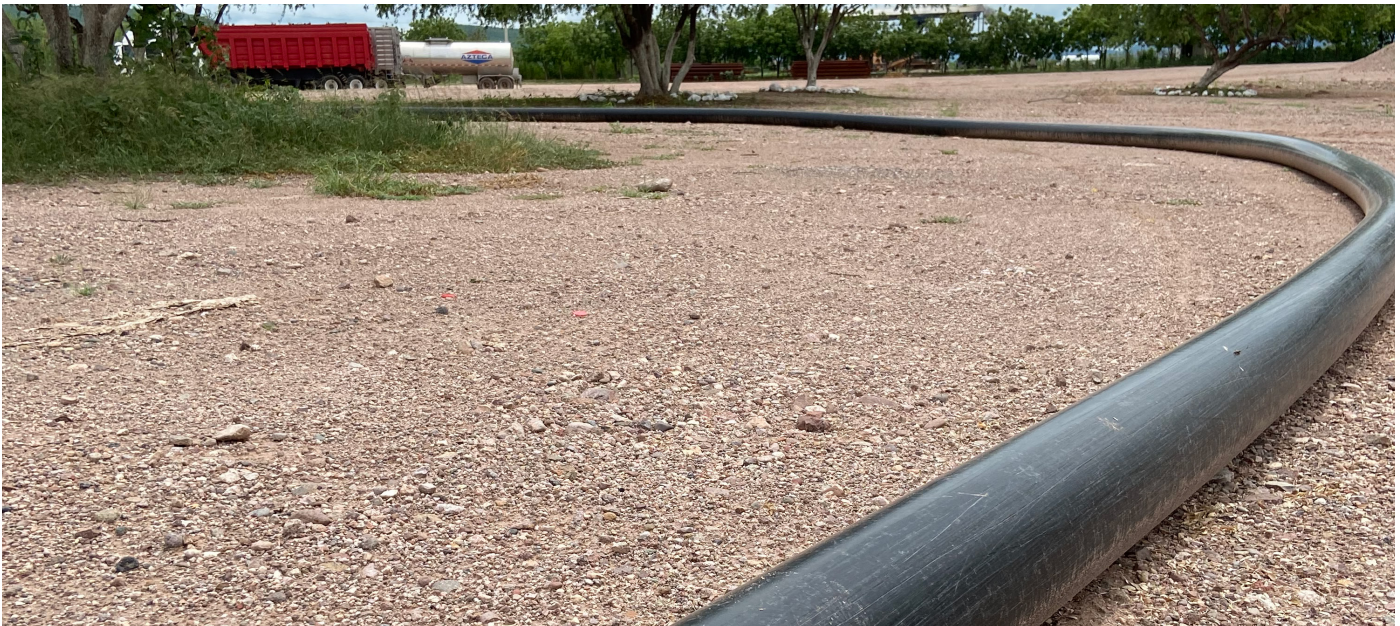
Pexgol pipe installation for the transport of water with solids (feathers, bones, viscera, etc.)
