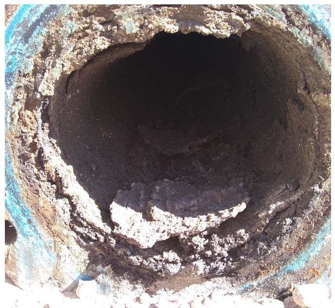
Embedded Carbon Steel Pipe
