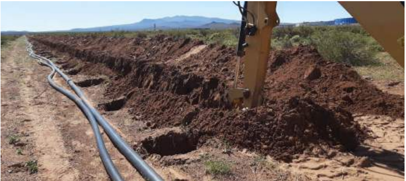
Dry gas line for pump activation.
