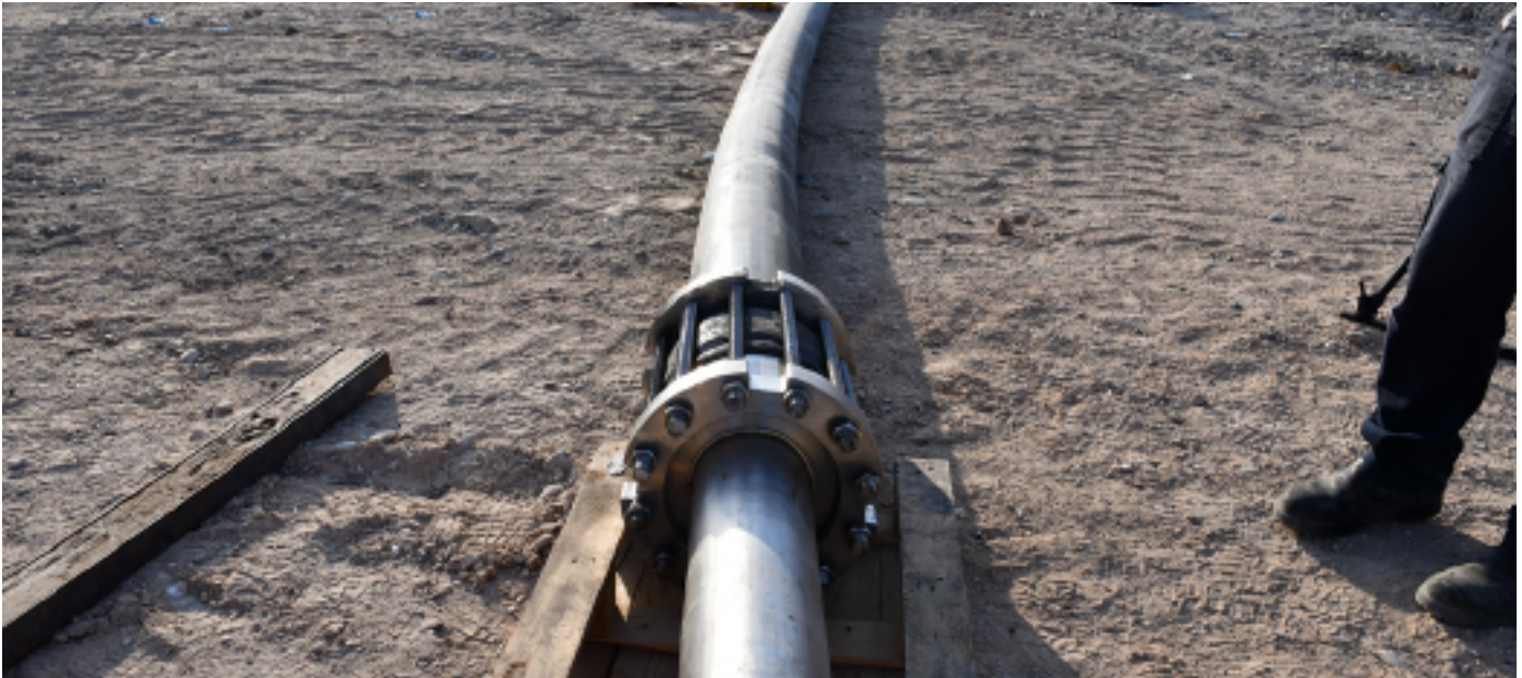
Installation of Pexgol pipe to transport brine at high pressure in a borehole.
