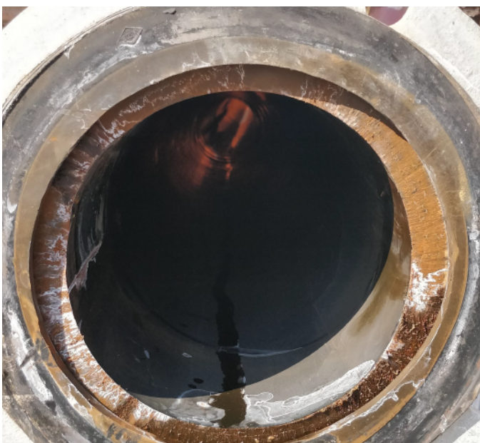
Test section installed in 2016, after two years there were no incrustations or leaks.
