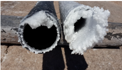
Suction from the pumps: Pexgol vs HDPE
